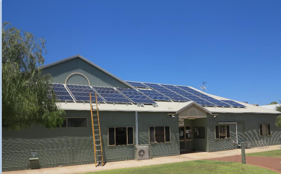
Coolgardie Recreational Centre solar PV installation
