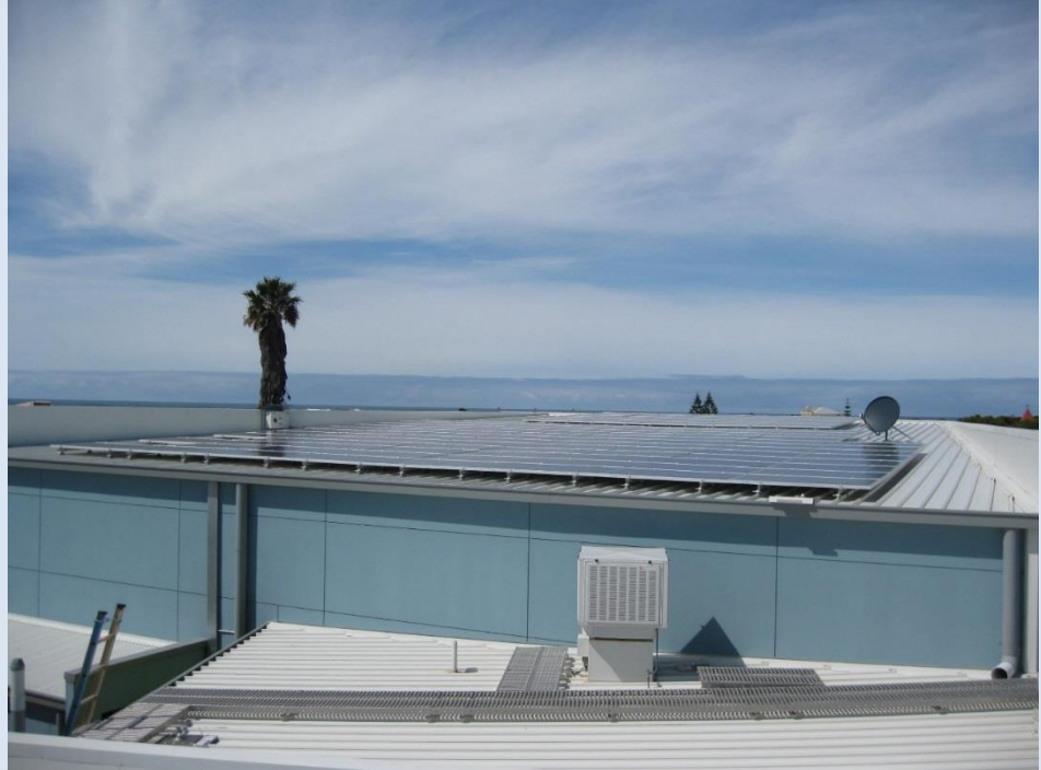
Shire of Ravensthorpe -Hopetoun solar PV installation
