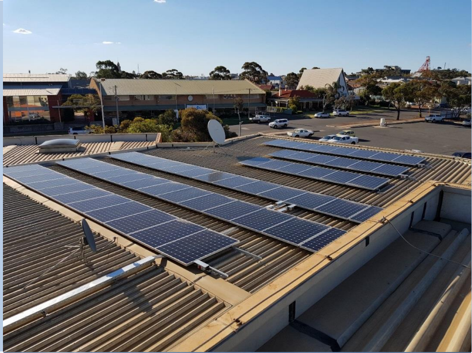
City of Kalgoorlie- Boulder Arts Centre solar- PV system
